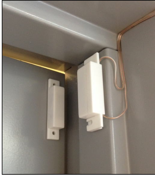
Figure 4-10 Open-Door Sensors Mounted to Door 48
